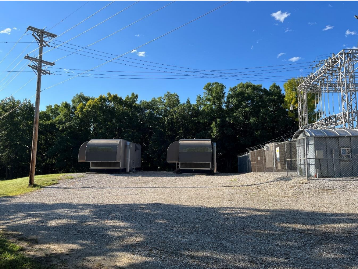
Substation 2, 1411 Noll Drive, Macon, MO 63552
